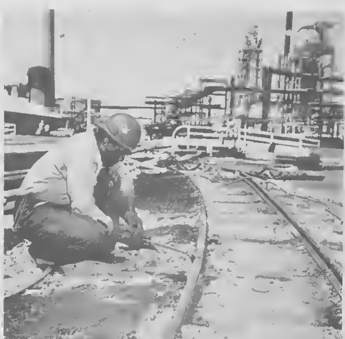
WELDER'S torch cuts once-shining rails into convenient lengths for scrapping. TORCH di weldet ta corta e riel den piezanan grandi pa worde bentá afor.
